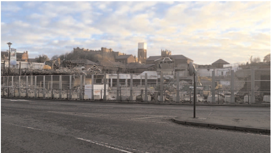
The demolition of the Gates Shopping Centre on Milburngate has opened up a new vistas of the Castle and Cathedral
